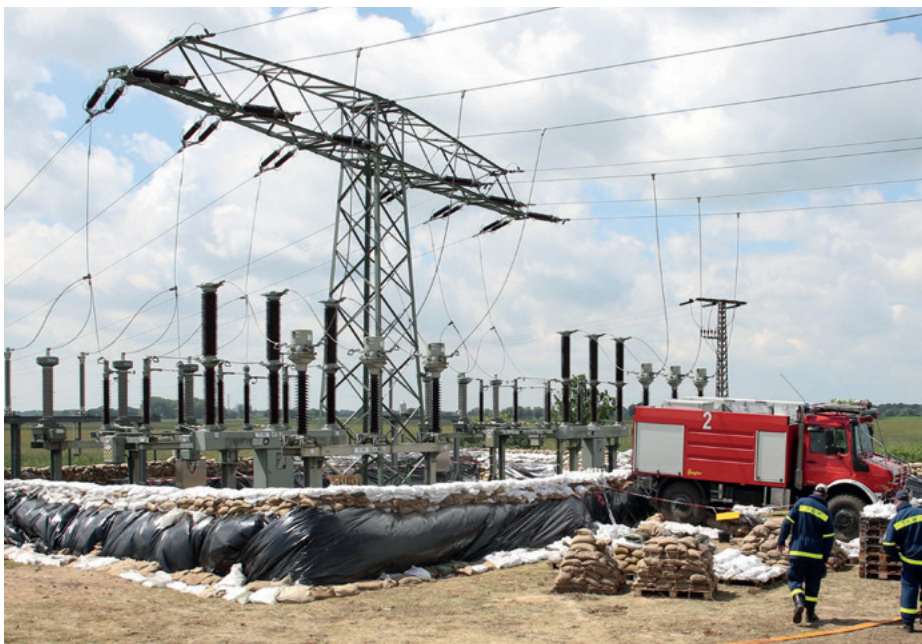
Flood damage near Stendal, Germany
