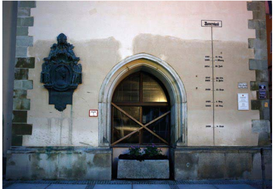
Even by historic standards, the June 2013 floods were extreme. Here the severe damage to Passau's City Hall can be compared with levels of previous major floods. (Photo: Michael Szönyi)
