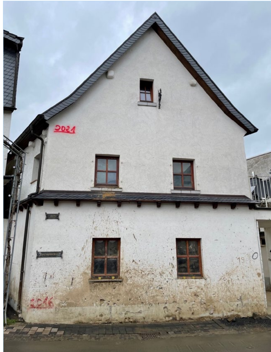
Flood markers at a central building in Dernau indicating the flood levels of 2016, 1910, 1804 and 2021 (bottom to top). Michael Szönyi, 5.4.2022.
